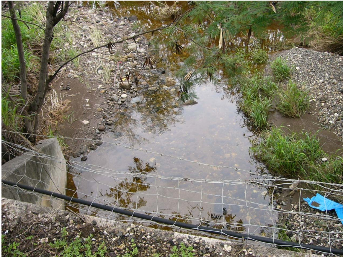
Outflow from culvert for Ulehawa Stream which runs under Lualualei Naval Access Road from the project site to the west (Mākaha) side of the road. Normally a dry streambed, this photo was taken immediately after the winter storm of December 11-14, 2008.
