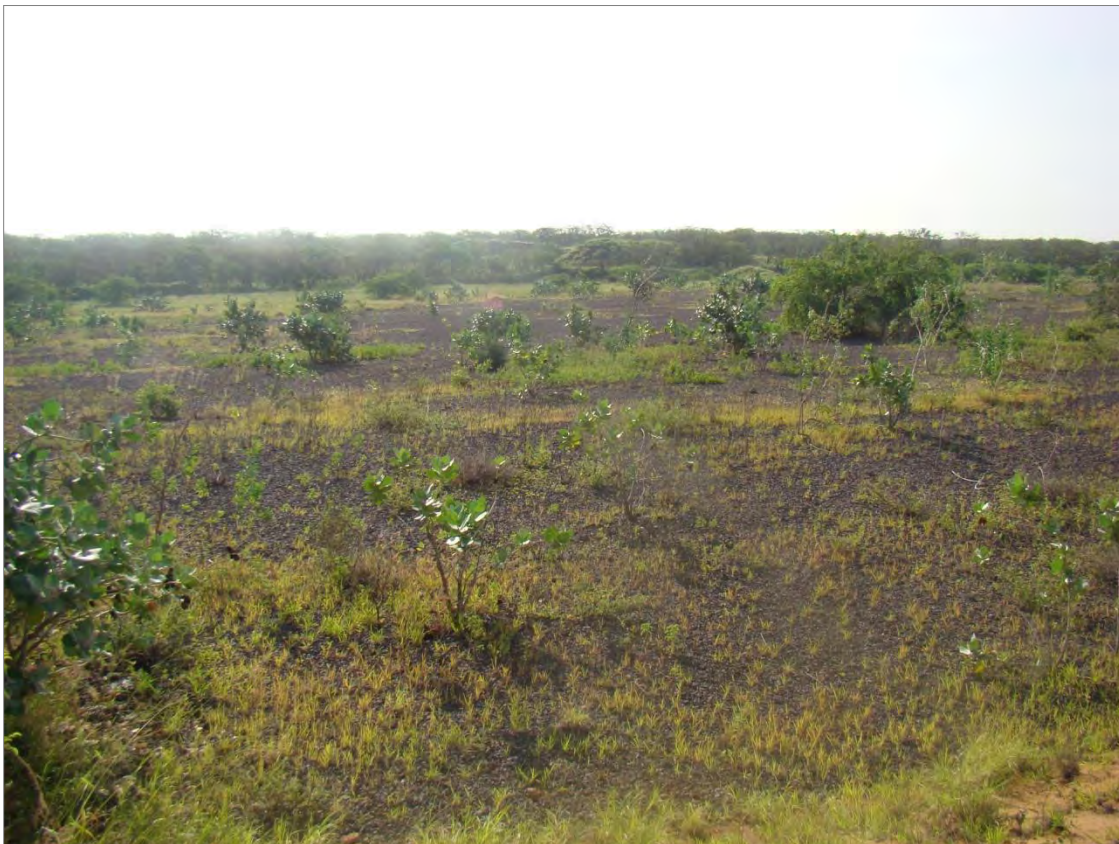
Figure 3 Area leveled from sand excavation and surfaced with a thin layer of gravel.
