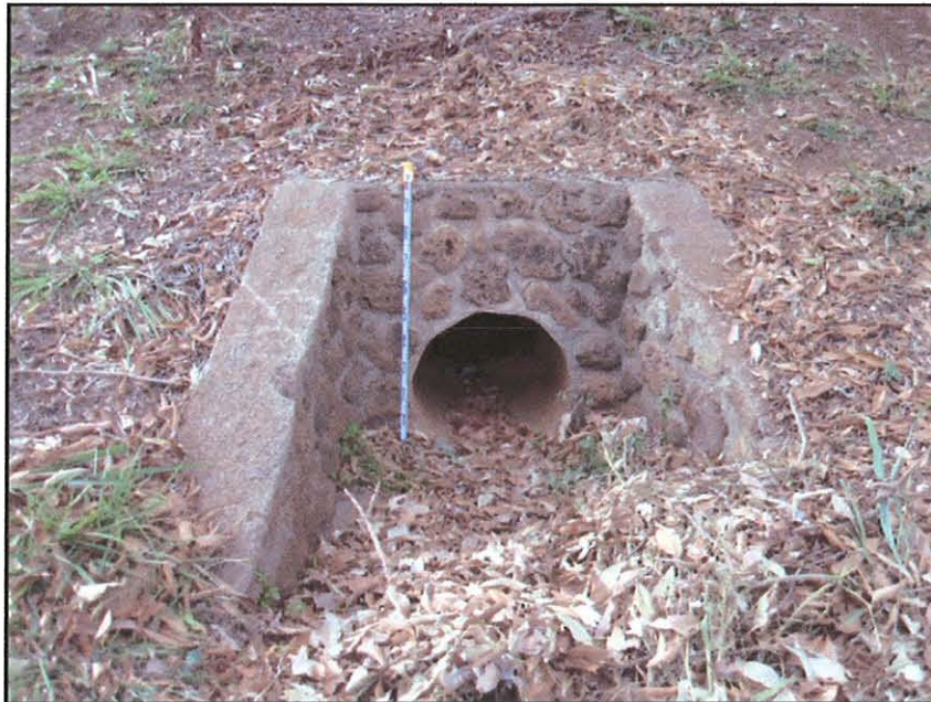
Figure 18. Modern culvert at the base of fill that comprises the ball park, view to north.
