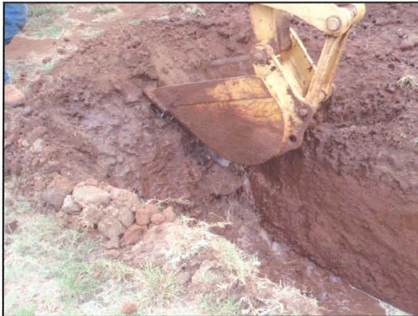
Figure 34. Backhoe Trench 1, showing the breach in irrigation water pipe, view to southeast.
