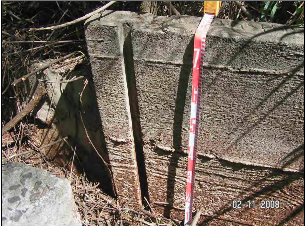
Figure 39. Photograph of sluce gate grooves observed at northern end of irrigation ditch, view to east
