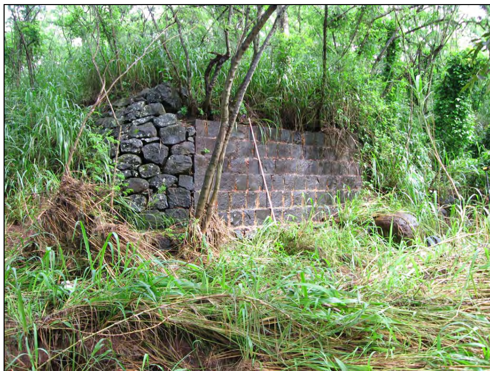
Figure 140. Photograph of SIHP # 50-80-09-9534 F bridge foundation/retaining wall on northern stream bank, view to northeast
