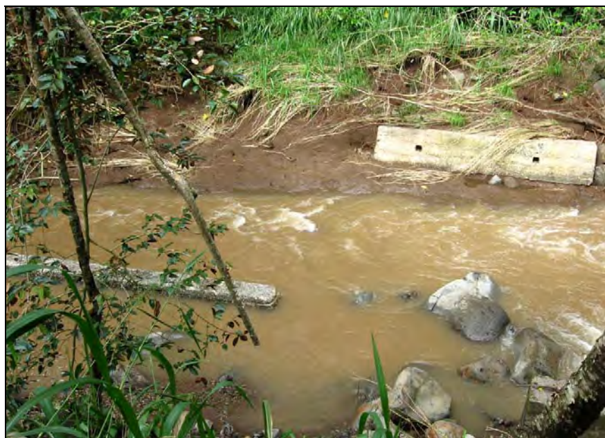
Figure 128. Photograph of SIHP # 50-80-09-9530 G reinforced concrete bridge foundations, western alignment, view to north
