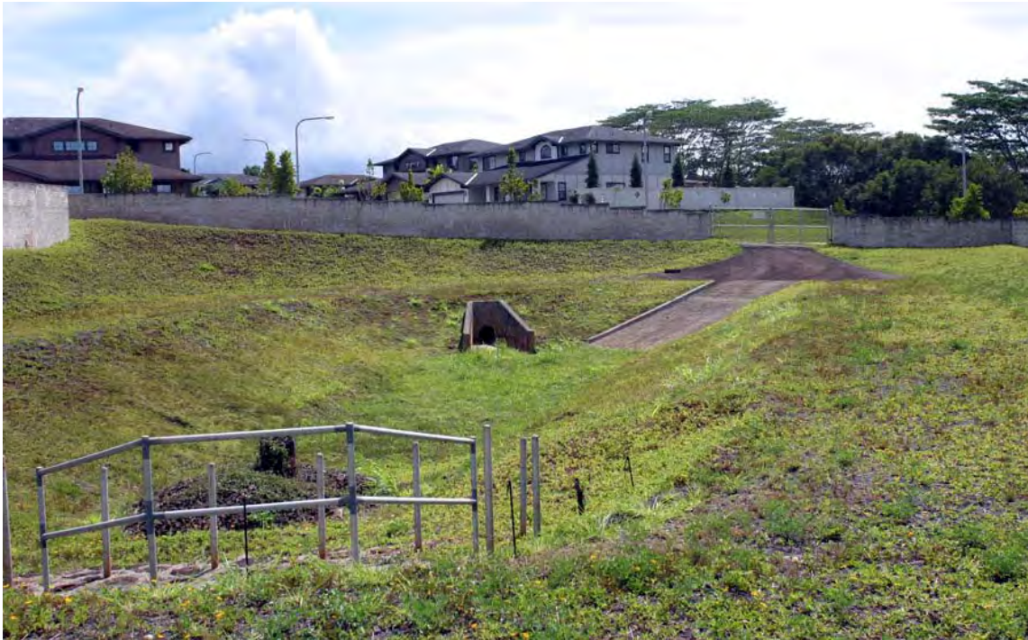
A small storm detention basin—example at Mililani Mauka Subdivision above Drain Line No. 2.
