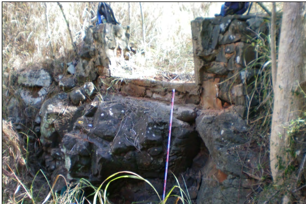
Figure 108. Photograph of SIHP # 50-80-09-9530 A irrigation ditch, showing flume support along eastern (upslope) edge of the ditch, view to north
