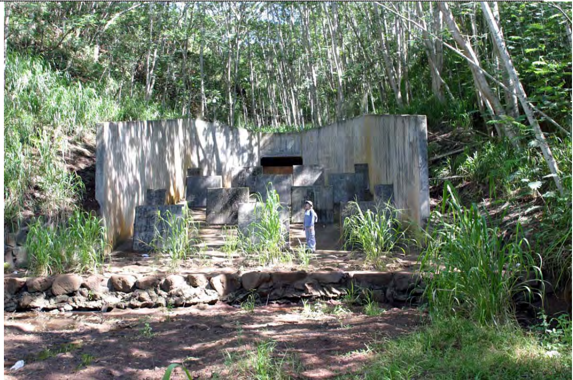
Figure 4. Drainage outlet (Mililani Mauka Drainline 2) into unnamed gulch upslope of proposed catchment basin (DB-2).
