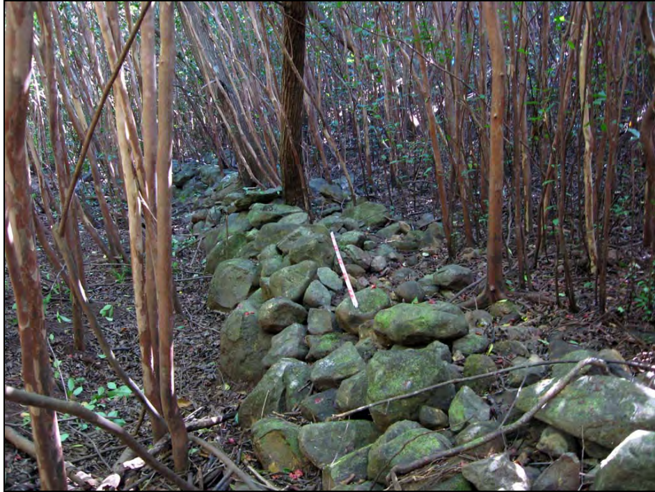
Figure 49. Photograph of SIHP # 50-80-09-7044 K stream channel improvements, showing mounded wall, view to south
