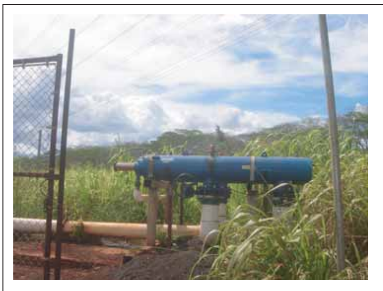
Photograph 8: Water Pump structure located on the north portion of the Subject Property.
