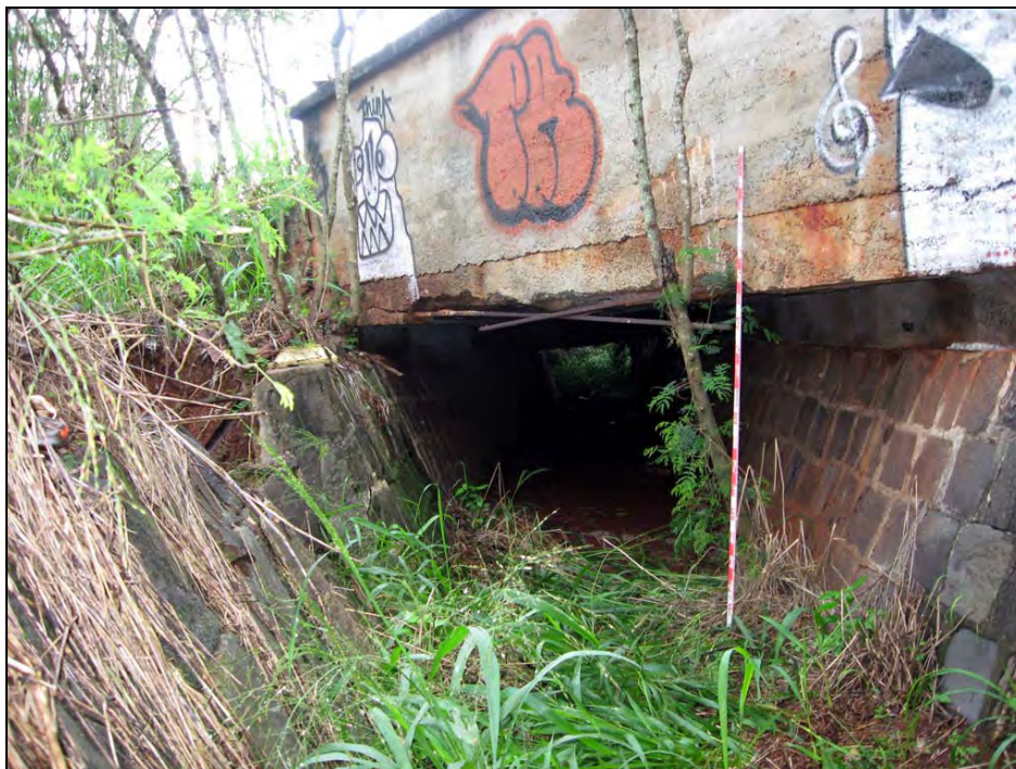
Figure 114. Photograph of concrete bridge over SIHP # 50-80-09-9530 A irrigation ditch, view to northeast
