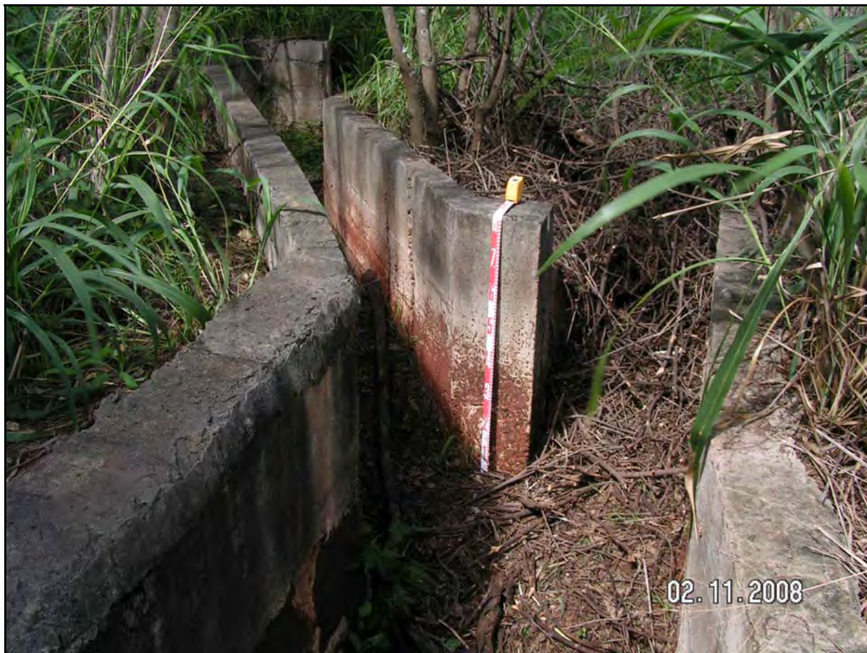
Figure 41. Photograph of concrete ditch leading to water control box (upper left had corner), view to north
