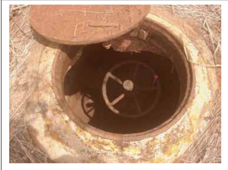
Photograph 7: Valve Pit (VP) 19 of the Hickam POL Pipeline.
