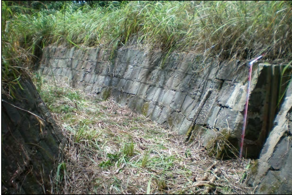
Figure 105. Photograph of SIHP# 50-80-09-9530 A irrigation ditch, showing cut basalt block lining, view to south
