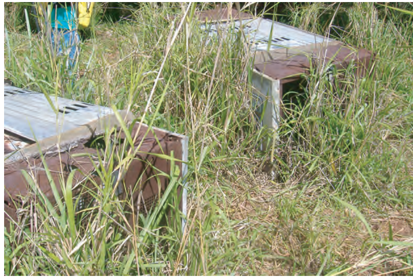
Photograph 13: Suspect transformers located on the central portion of the Subject Property.
