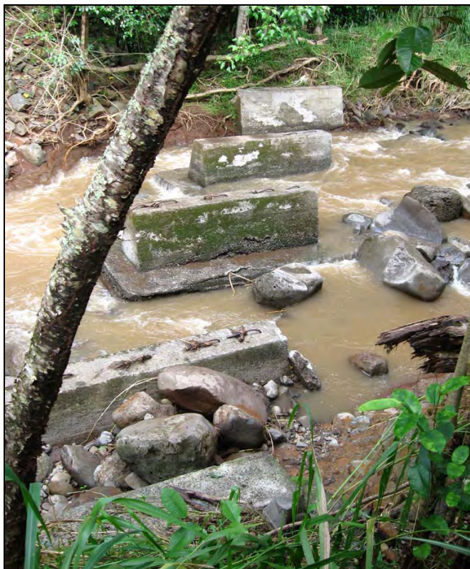
Figure 127. Photograph of SIHP # 50-80-09-9530 G reinforced concrete bridge foundations, eastern alignment, view to northeast
