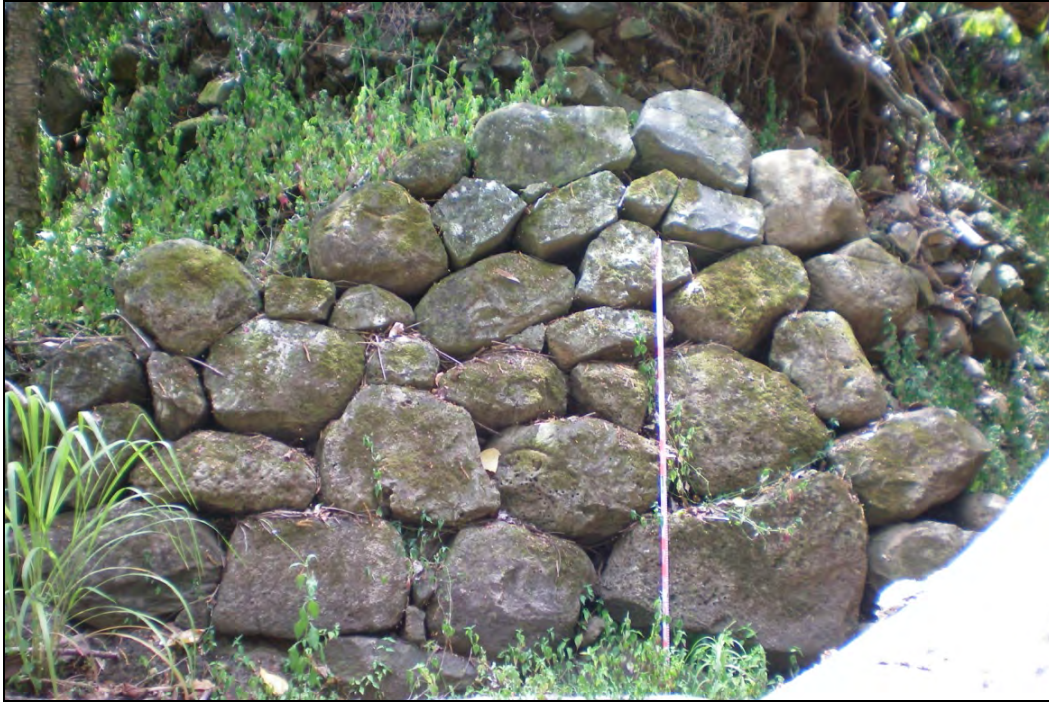
Figure 129. Photograph of SIHP# 50-80-09-9530 G stacked-stone retaining wall along stream bank, view to south
