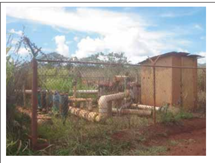
Photograph 9: Northernmost water pump structure located on the north portion of the Subject Property.
