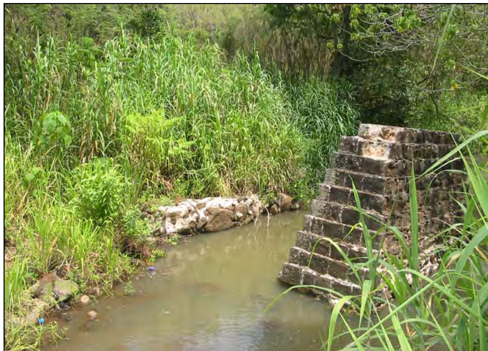
Figure 139. Photograph of SIHP # 50-80-09-9534 F bridge foundations with the Kīpapa Stream channel, view to east
