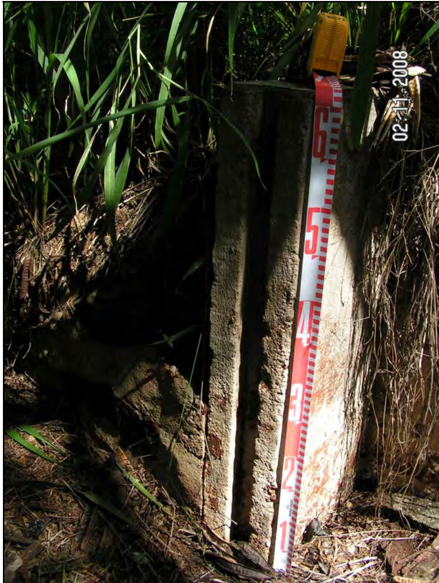
Figure 40. Photograph of a water control gate at the end of the west branch of SIHP # 50-80-09-6959, facing southeast
