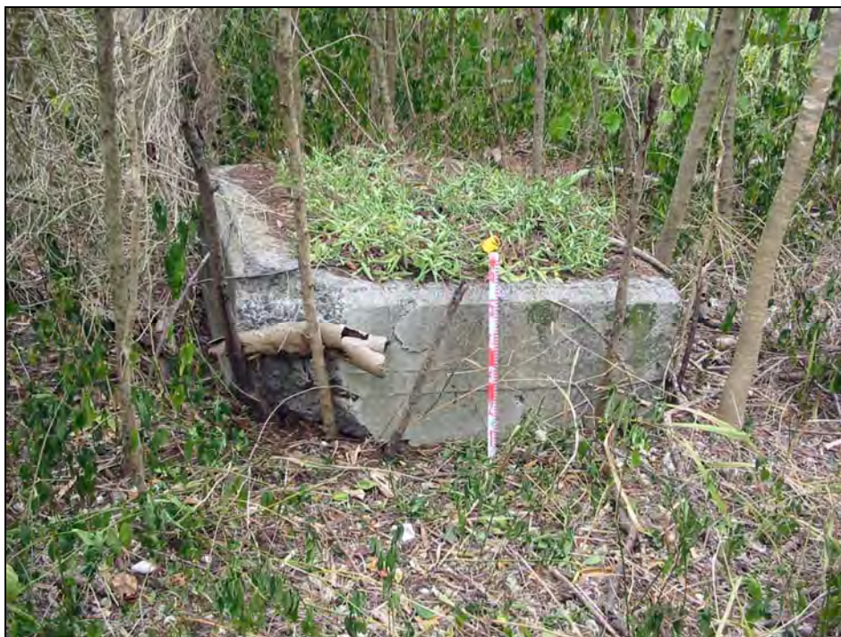
Figure 123. Photograph of concrete foundation adjacent to SIHP # 50-80-09-9530 F railroad berm, view to southwest
