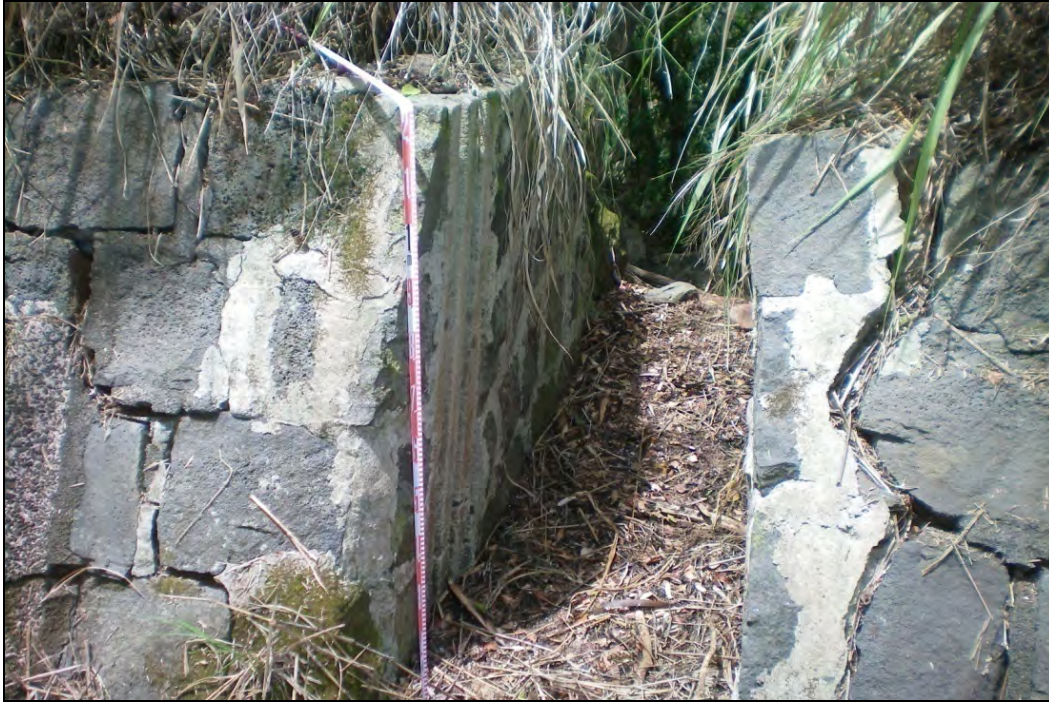
Figure 107. Photograph of SIHP # 50-80-09-9530 A irrigation ditch, showing sluice gate along western (down slope) edge of the ditch, view to west
