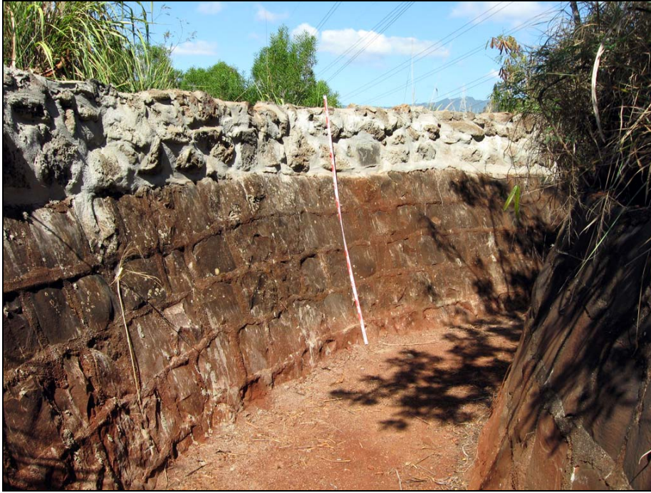
Figure 9. SIHP # 50-80-09-9530 Feature A irrigation ditch, showing recently constructed stone and mortar lining above the cut basalt block and mortar ditch lining (view to southwest)
