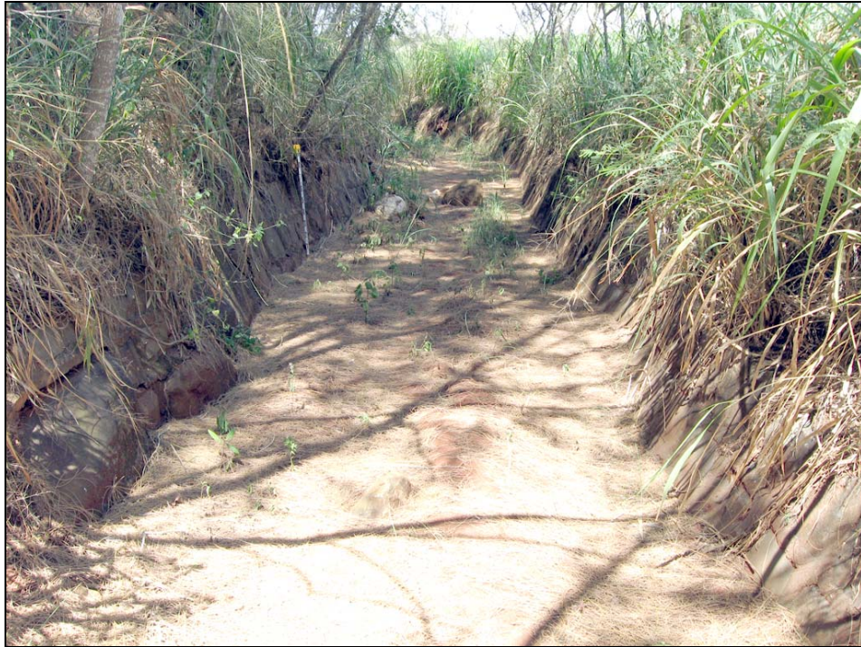
Figure 27. SIHP # 50-80-09-9530 Feature A irrigation ditch, showing portion of the ditch partially filled with sediment (view to southwest)
