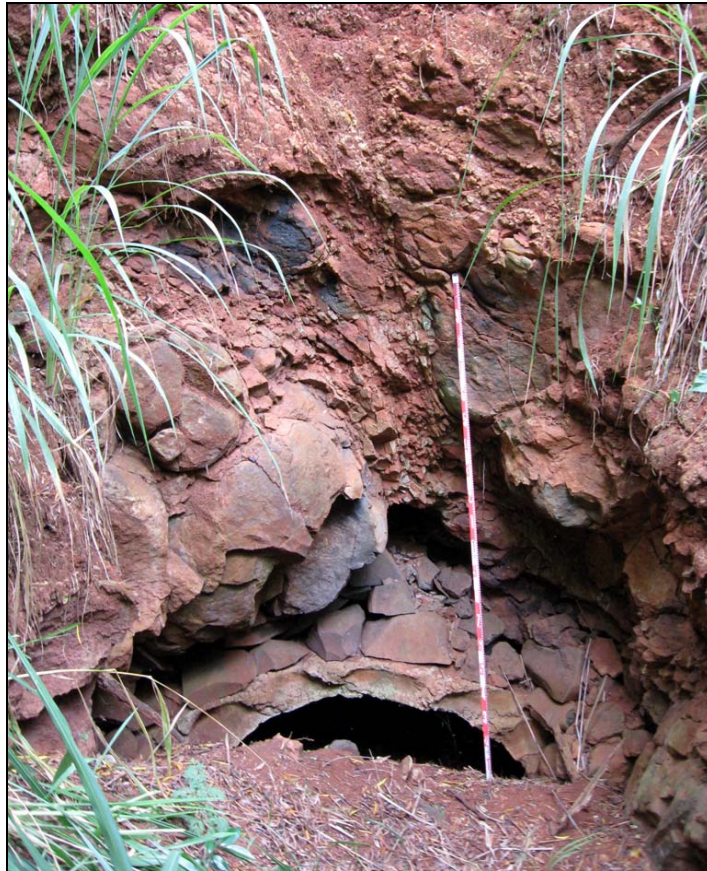
Figure 32. Photograph of a collapsed portion of the SIHP # # 50-80-09-9530 Feature A ditch tunnel
