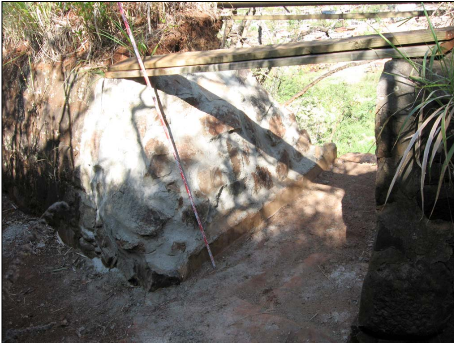
Figure 10. SIHP # 50-80-09-9530 Feature A irrigation ditch, showing recent modifications to the sluice gate and ditch outlet at the edge of Kīpapa Gulch (view to southwest)
