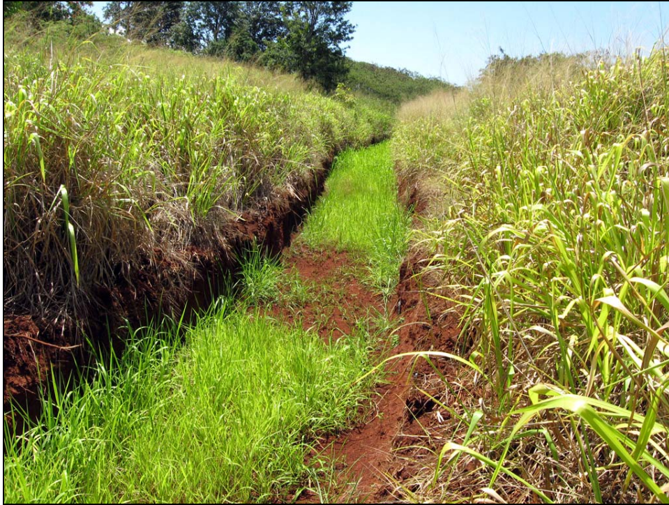
Figure 11. Recently constructed drainage ditch along the edge of the tablelands, upslope of the SIHP # 50-80-09-9530 Feature A irrigation ditch
