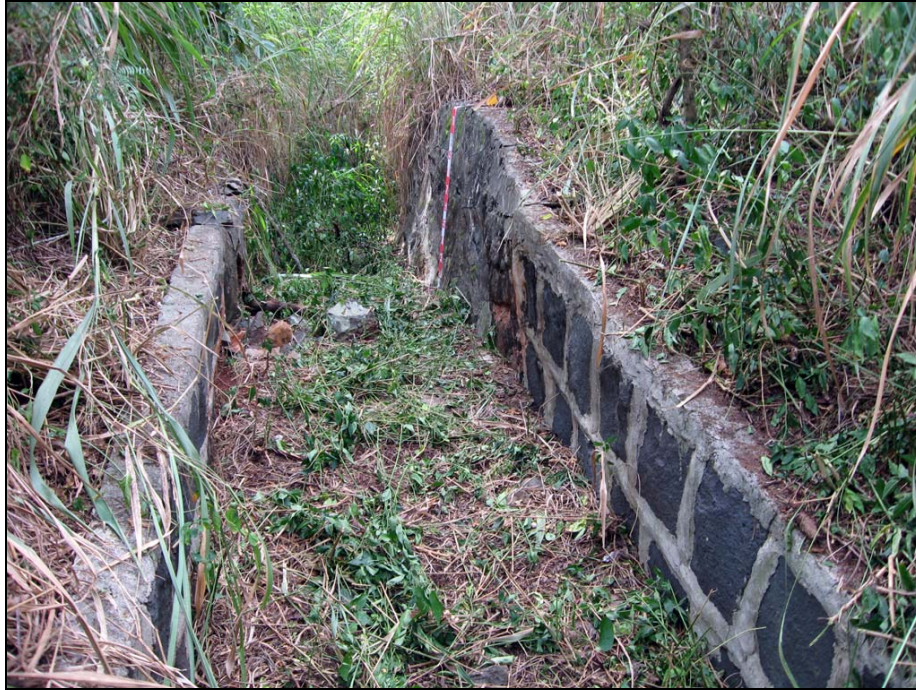
Figure 34. Photograph of SIHP # 50-80-09-9530 Feature B ditch, showing cut (“dressed”) stone and mortar construction transitioning to natural stone and mortar construction, view to southeast
