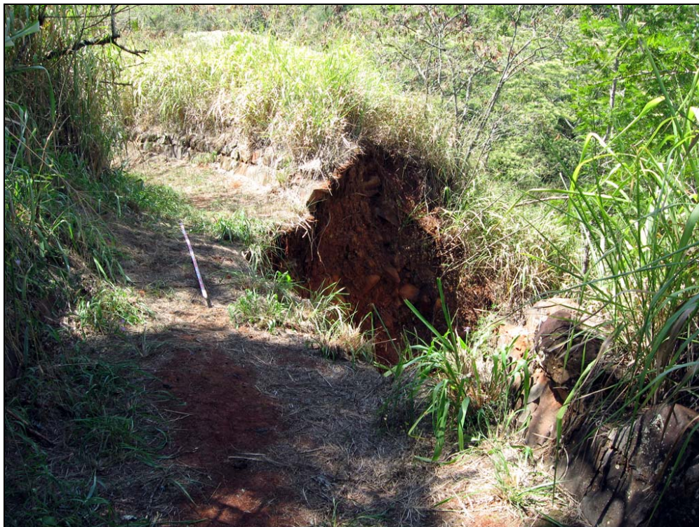
Figure 28. SIHP # 50-80-09-9530 Feature A irrigation ditch, showing portions of the ditch damaged by flooding
