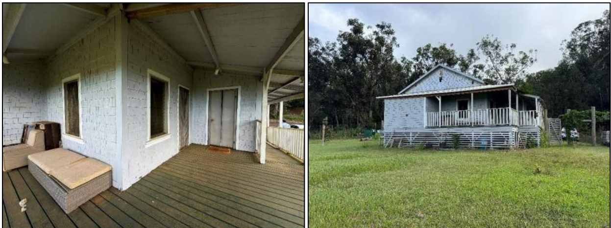
Figure 52. Lanai that wraps around Structure D's southwest and southeast facades (left) and the southwest and southeast facades of Structure D (MASON, 2024).
