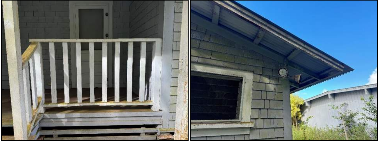
Figure 33. Details of Structure C's rear (northeast) facade, including the rear lanai railing (left), window casing, and exposed rafter and purlins (right) (MASON, 2024).
