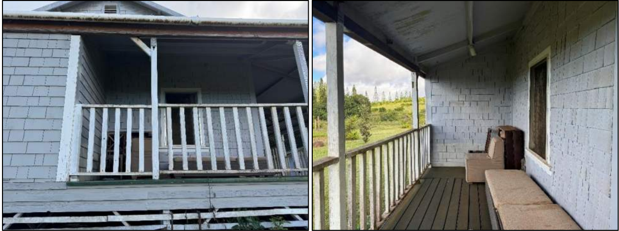
Figure 47. Details of Structure D's front (southwest) facade, including shingle siding, wraparound lanai, front storage room, and wood lanai features (MASON, 2024).
