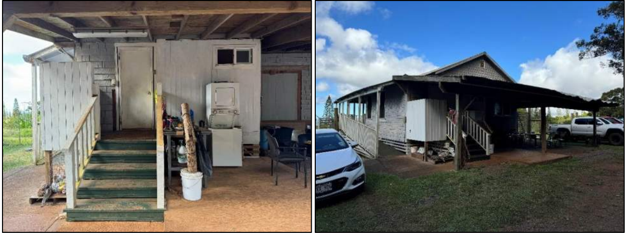
Figure 50. Structure D's northeast facade (left) and northeast and southeast facades (right) (MASON, 2024).
