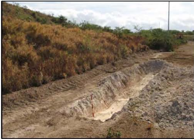
Test Trench 51 at south end of Stockpile 1, showing previously disturbed karst bedrock (view to east).
