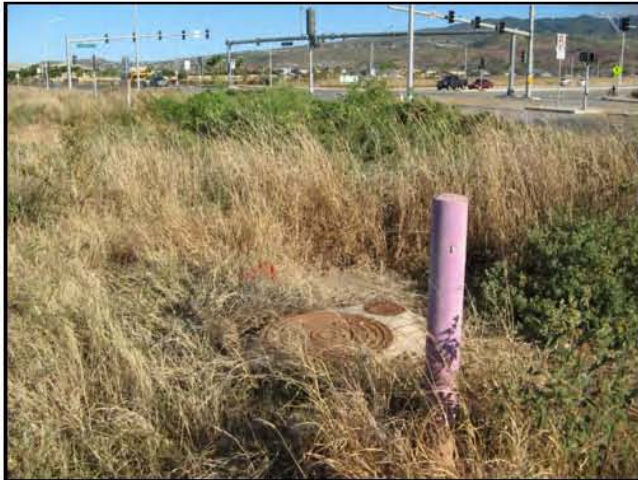
Another reclaimed water manhole near northeast corner of project area (view to northwest).
