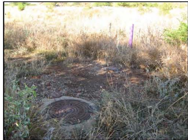
Existing utility manhole (Reclaimed water) located ca. 10 m west of the old plantation dirt road in NE Quad. (runs roughly parallel to dirt road), purple bollards in background (view to west).
