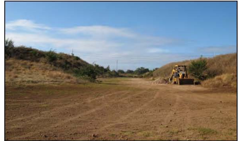
Excavating Test Trench 49 between Stockpiles 1 and 2, on edge of Stockpile 2 (view to south).
