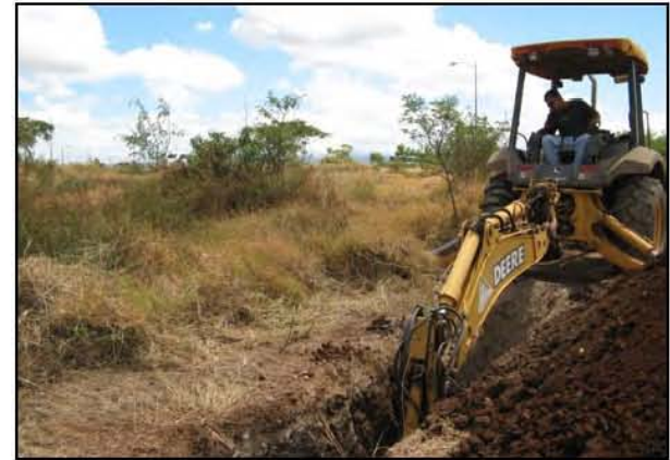
Test Trench 18, excavating from west to east (note cars in background are on Kapolei Pkwy. (view to northeast).
