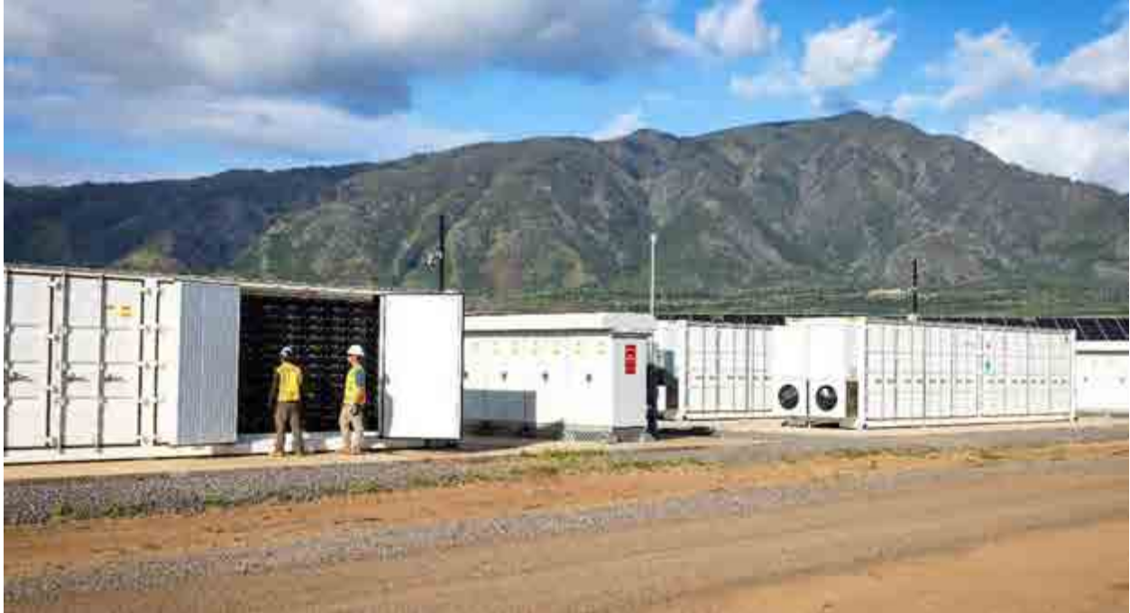
Photograph of typical power conversion station including battery energy storage system and associated components ( Kūihelani Solar + Storage )
