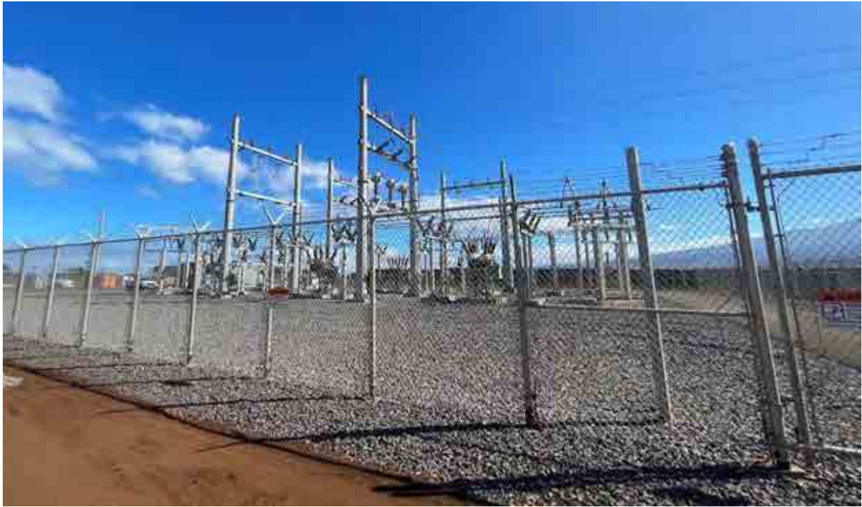
Photograph of typical switchyard ( Kūihelani Solar + Storage )
