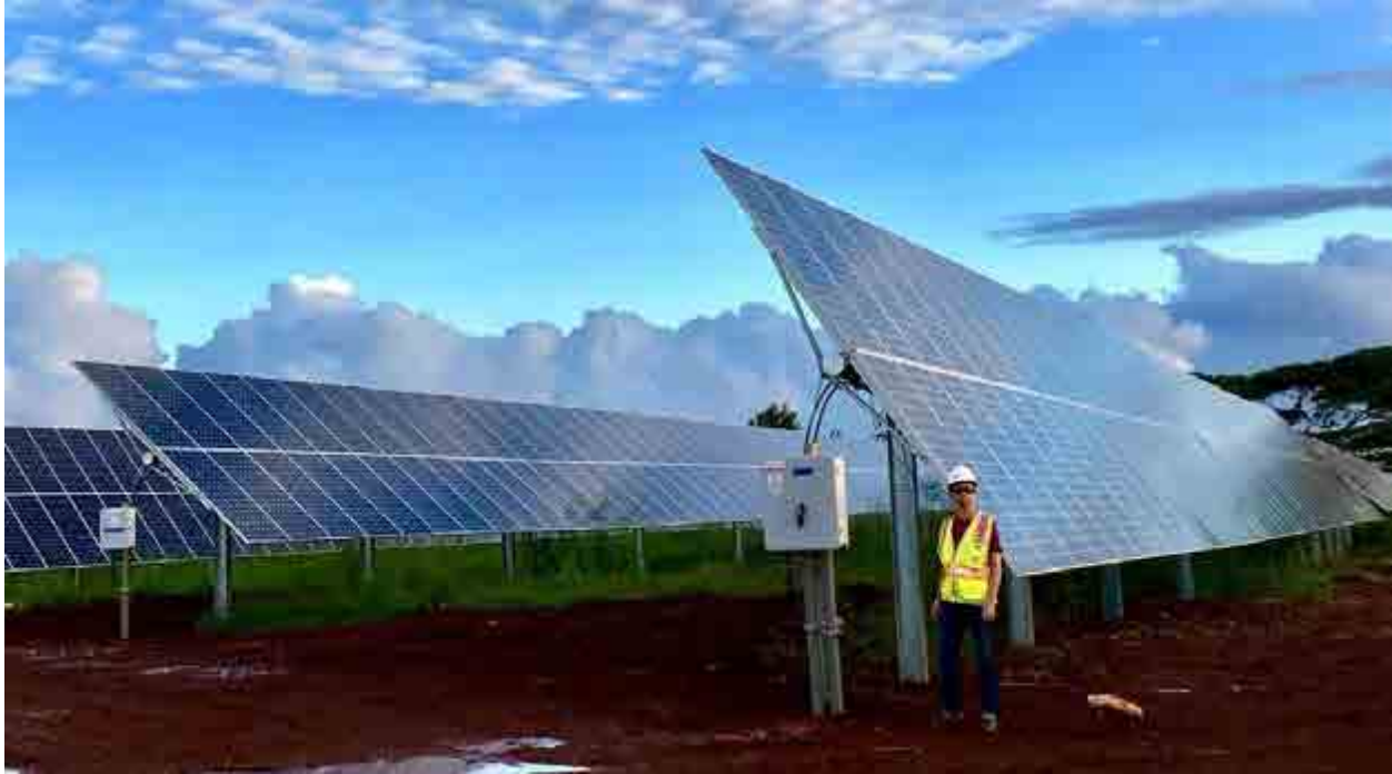
Photograph of typical solar photovoltaic modules on single-axis tracking system ( Lawai Solar Project )
