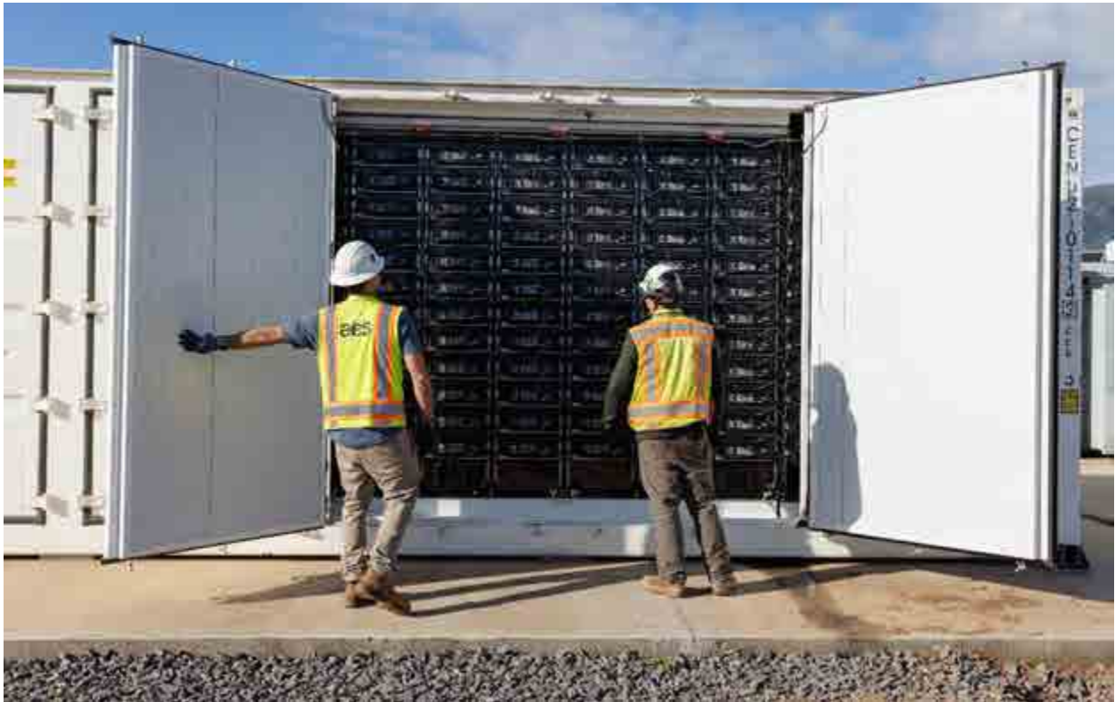
Photograph of typical battery racks within storage container ( Kūihelani Solar + Storage )
