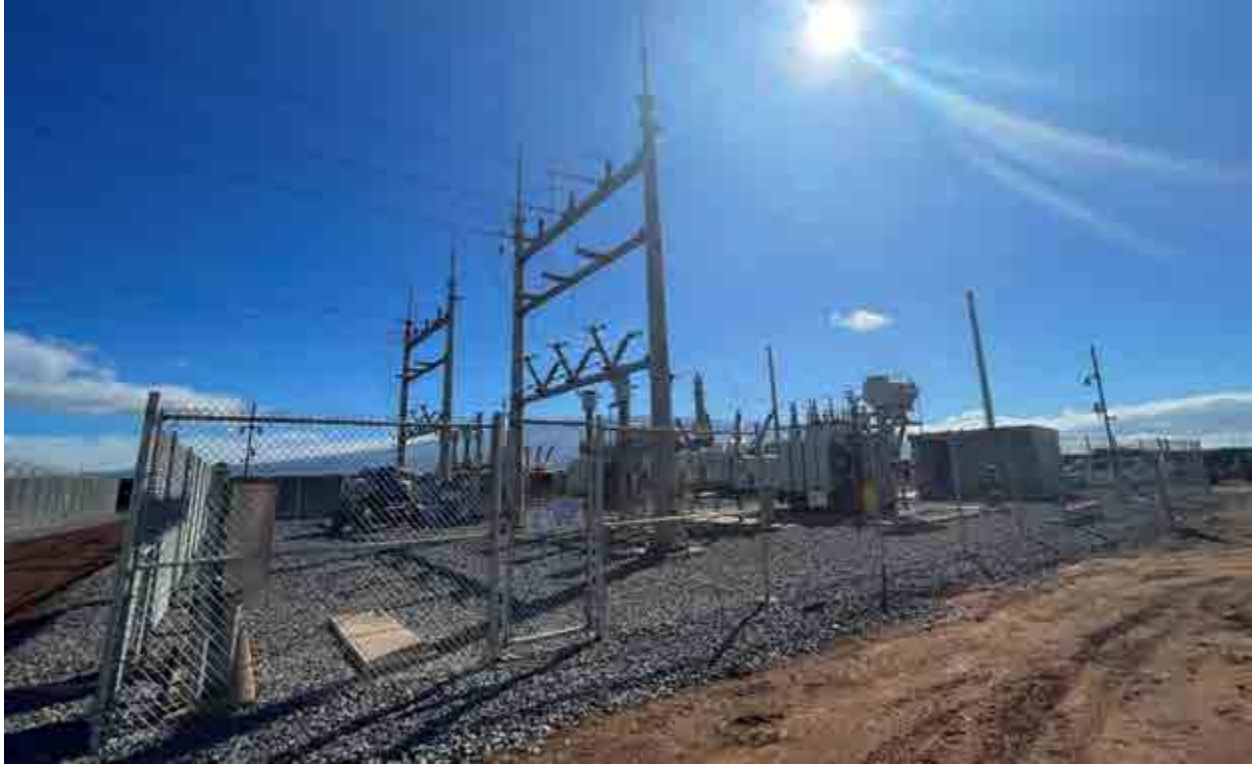
Photograph of typical Project substation ( Kūihelani Solar + Storage )
