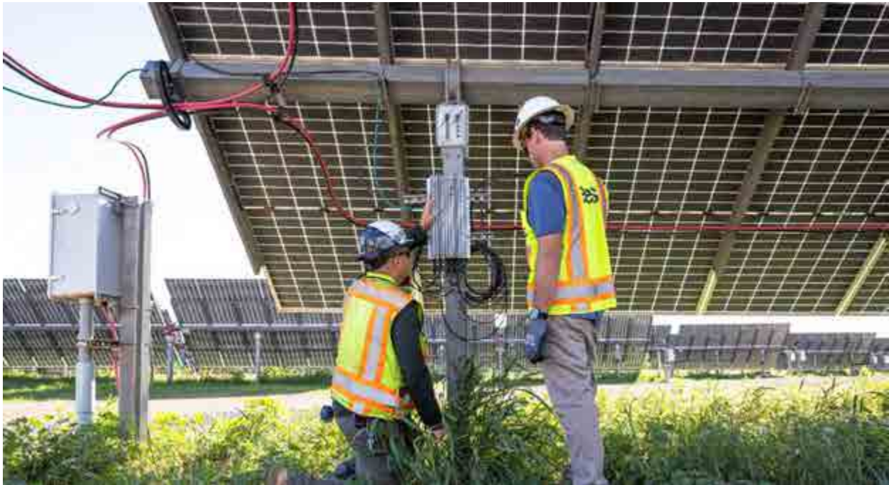
Photograph of typical DC collection cabling system and disconnect switch stations ( Kūihelani Solar + Storage )
